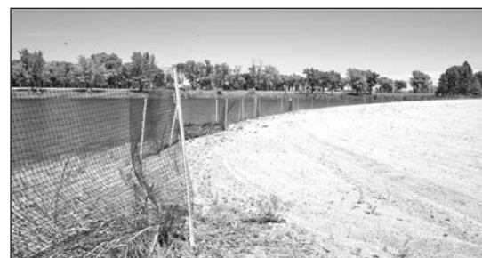
A fence with light netting has been placed along the water's edge at Chief Red Robe Park and the swimming beach.
