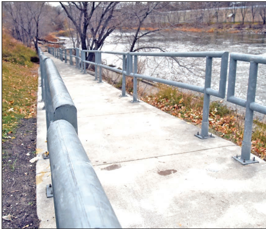
There was considerable damage to the ramp, and metal railings that provides citizens an opportunity to fish just below the dam in Thief River Falls. The city is hoping that funding from FEMA will help bring the handicapped-accessible ramp that provides access to fishing below the dam into compliance, and that the city will receive financial assistance for the work already completed. FEMA officials toured several sites within the community.
