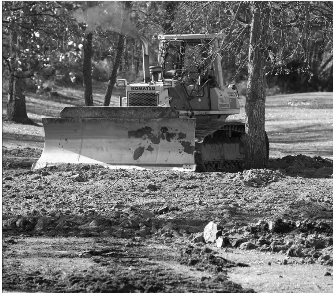
Dirt is packed on the 18th fairway at the Thief River Golf Club near the previous location of the cart paths. The 18th fairway has been prone to flooding since the back nine holes were added at the Thief River Golf Club in 1994. It will be raised an average of four feet to get the fairway above flood stage.
