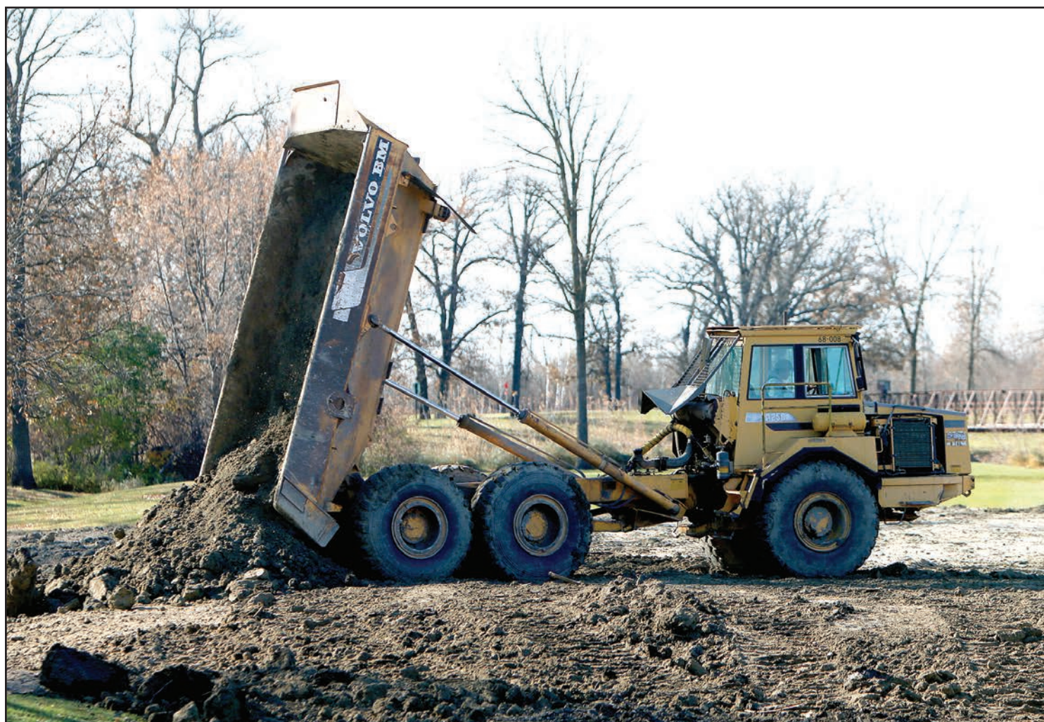
The 18th hole at the Thief River Golf Club will look quite a bit next year after work was done this fall to raise the fairway above minor flood stage. Dirt was removed from an area adjacent to the 18th fairway, loaded into dump trucks and dumped on the fairway where it was leveled and packed by bulldozer.
