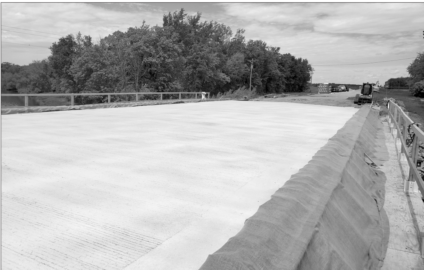
The deck was poured Friday, June 7 for the new Kratka bridge in rural Pennington County. Pennington County Engineer Mike Flaagan told the Pennington County Board that the next steps include the approach panels on each side of the bridge, grading, and installing the rails. Redstone Construction LLC is replacing the County State
