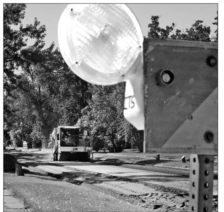
Construction crews started work on Kendall Avenue from First to Third Street, and Crocker Avenue from First to Mussey last week. This is part of the 2024 Streets and Utilities Improvement project in Thief River Falls. Part of the project involves widening Kendall Avenue, which is why so many trees were removed. Davidson Construction had the low bid of $1,267,480.50. The bid was within 8% of the engineer's estimate of $1,174,992. Please note that the City of Thief River Falls also has planned a reconstruction project along First Street from the railroad tracks west of Conley Avenue to Highway 59; however, the city is receiving federal funding for that project. Bids for the project have not been considered yet.
